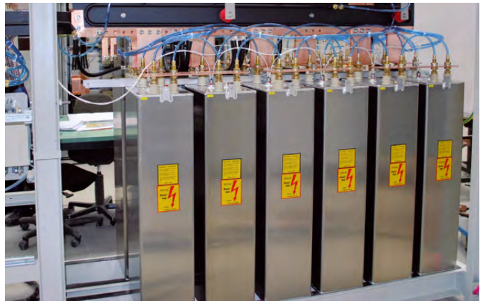
Power electronics with water chiller
